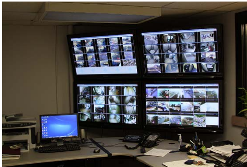
Central Security Dispatch Monitor Station
