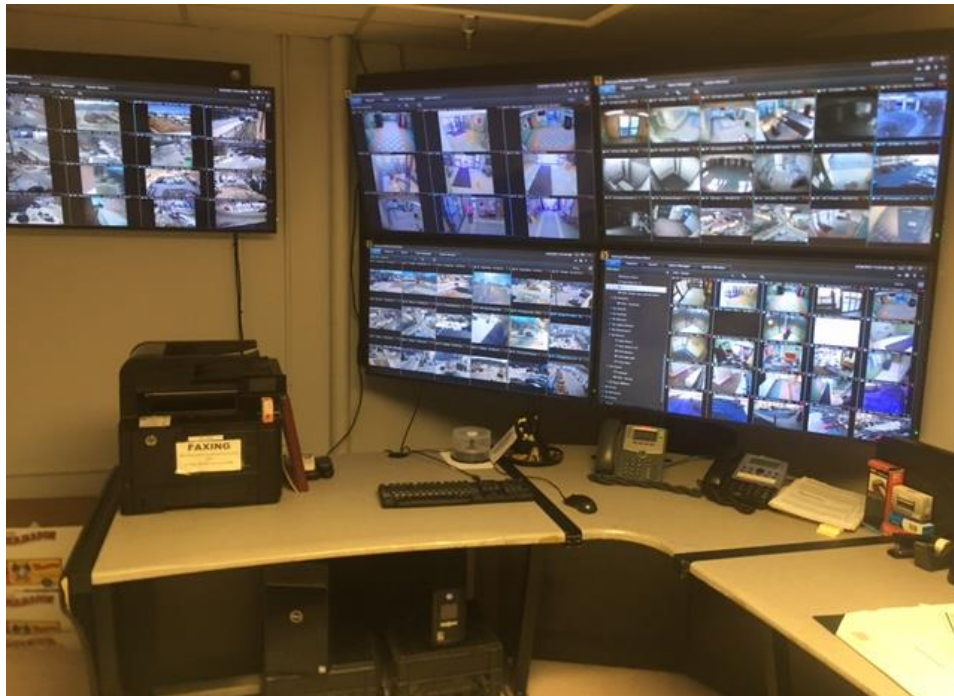
Central Security Dispatch Monitor Station
